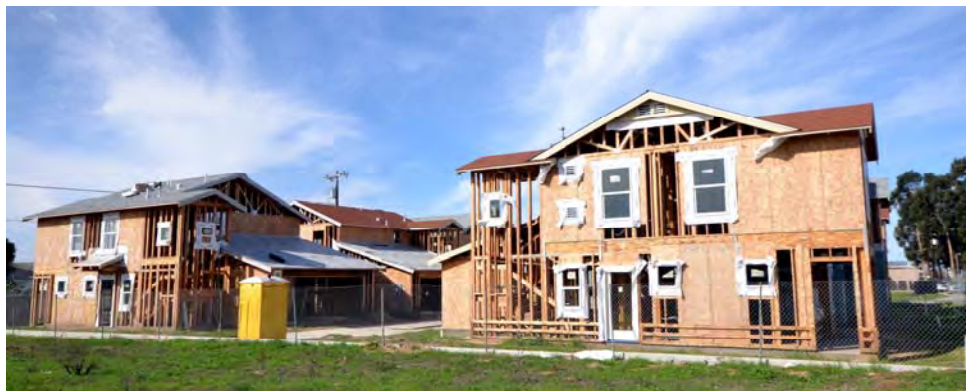
Self-help homes under construction in Oceano in mid-March. The buyers' construction labor reduces the required down payment. Completion is expected by August.
