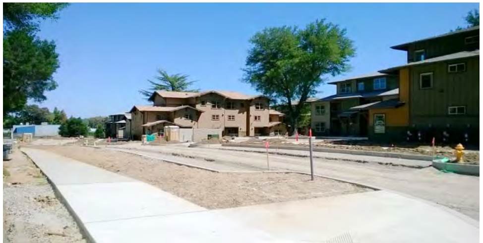
Phase 1 of the Oak Park redevelopment project in Paso Robles is nearing completion. Phase 2 will continue with the same design and have 69 additional units. Eventually, Oak Park will have over 300 new rental homes.
