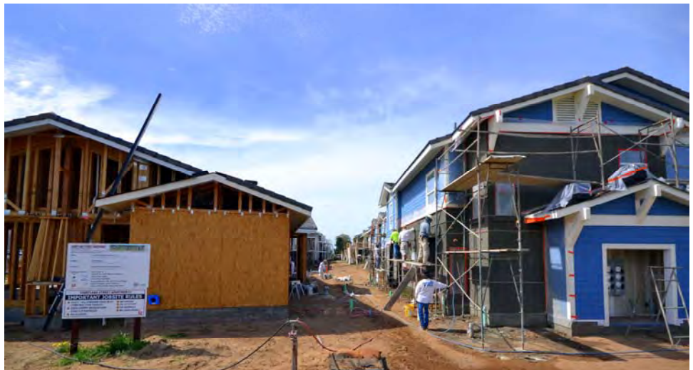
Courtland Street Family Apartments under construction in Arroyo Grande in mid-March. The units will be completed in August.
